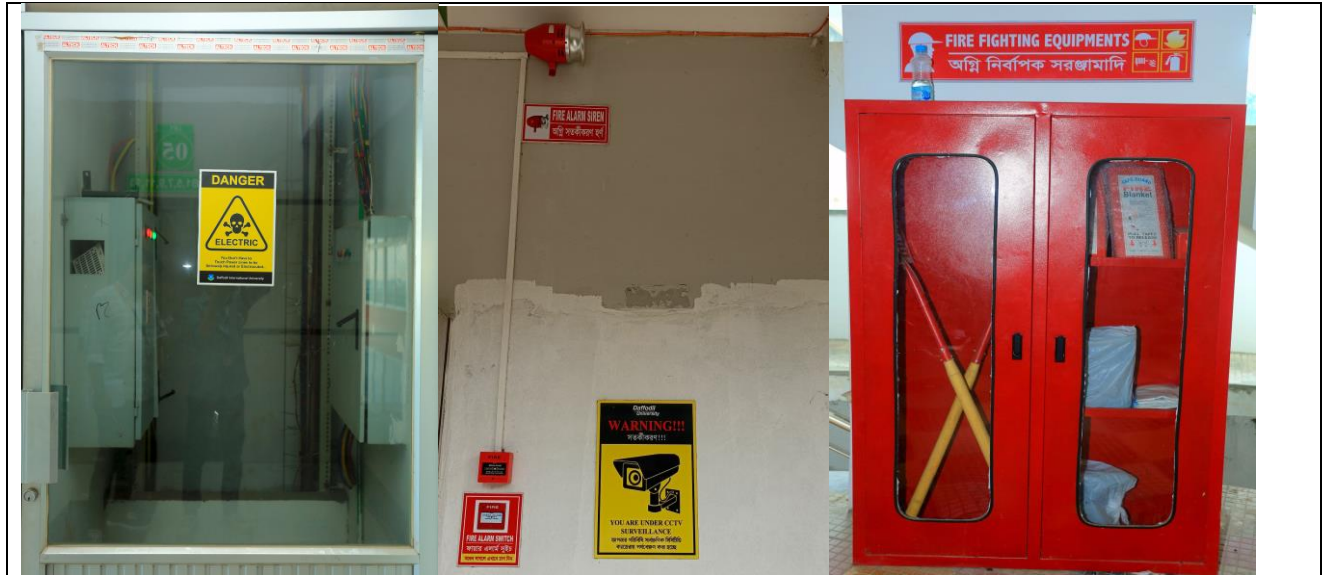
Secured Energy monitoring area; Automatic fire alarm system and firefighting equipment
