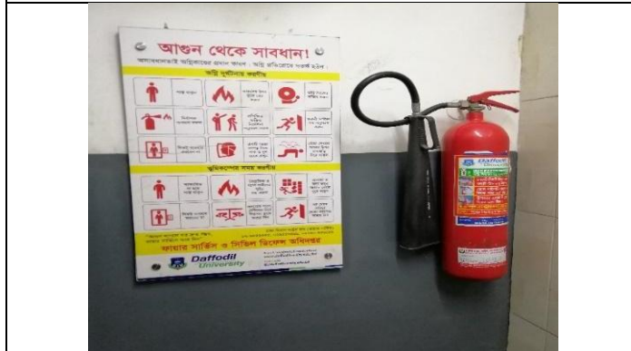
Fire Extinguisher along with Instructions to be followed (in local language)
